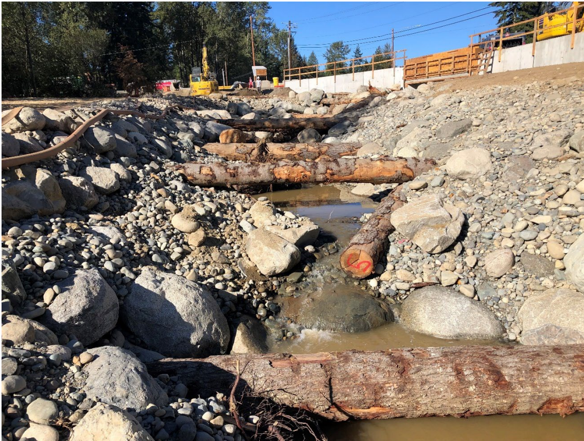
Image taken from a project in Centennial Creek, Snohomish County. This was a fish passage barrier correction.
