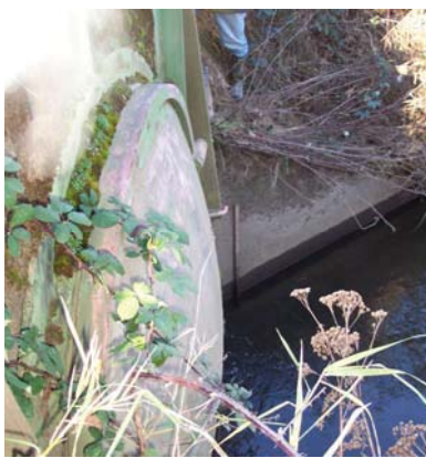
This flap gate prevents high flows in the Green River from entering Gilliam Creek
