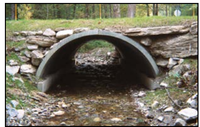
The MDT evaluated bottomless culverts as an option to improve stream function and provide wildlife passage.
