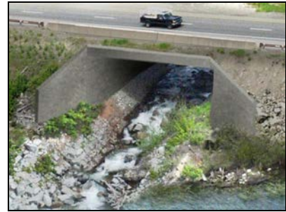
The MDT considered mid-sized stream crossings to allow a wider area for natural stream function and wildlife movement. (Design Visualization)
